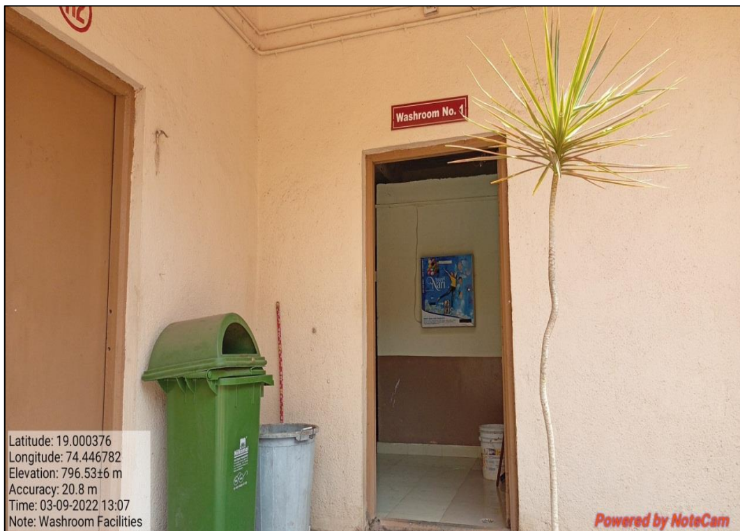
Picture 16: Washroom Facilities for Ladies at Rajmata Jijau Girl's hostel
