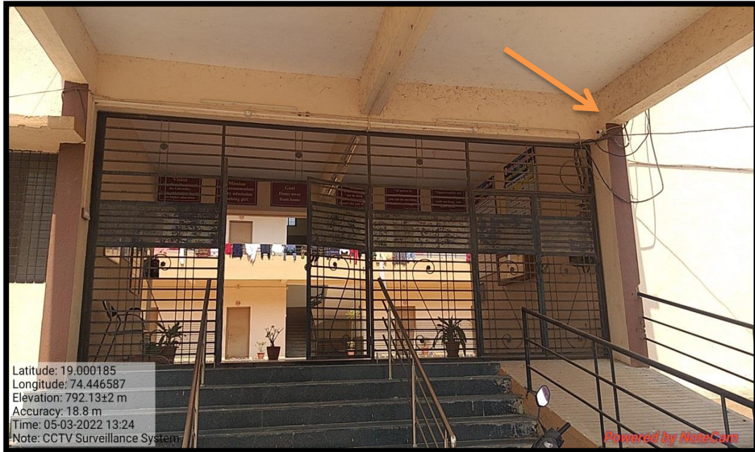
Picture 1: CCTV Surveillance System at Rajmata Jijau Girl's hostel
