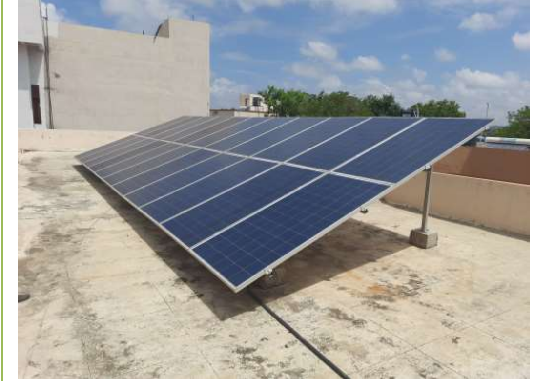
Solar Photovoltaic System- 7.2kWp- Girl's Hostel
