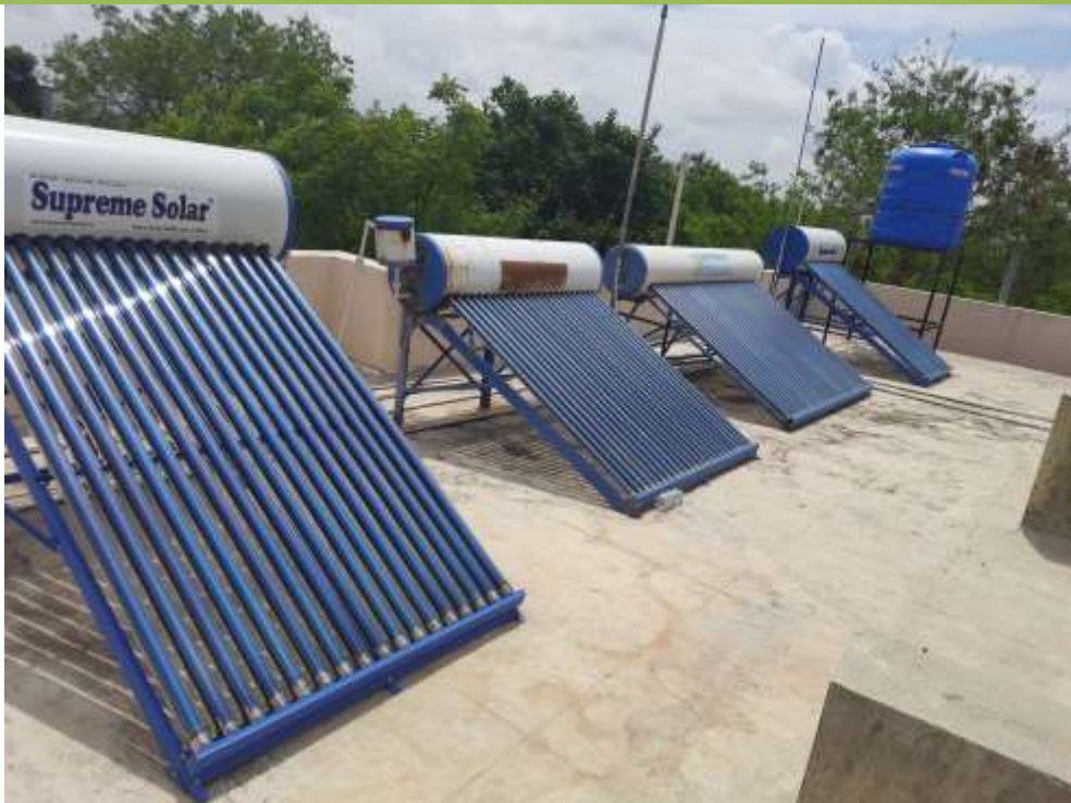
Total Solar Water Heating System- 2760litres/day- Girl's and Boy's Hostel
