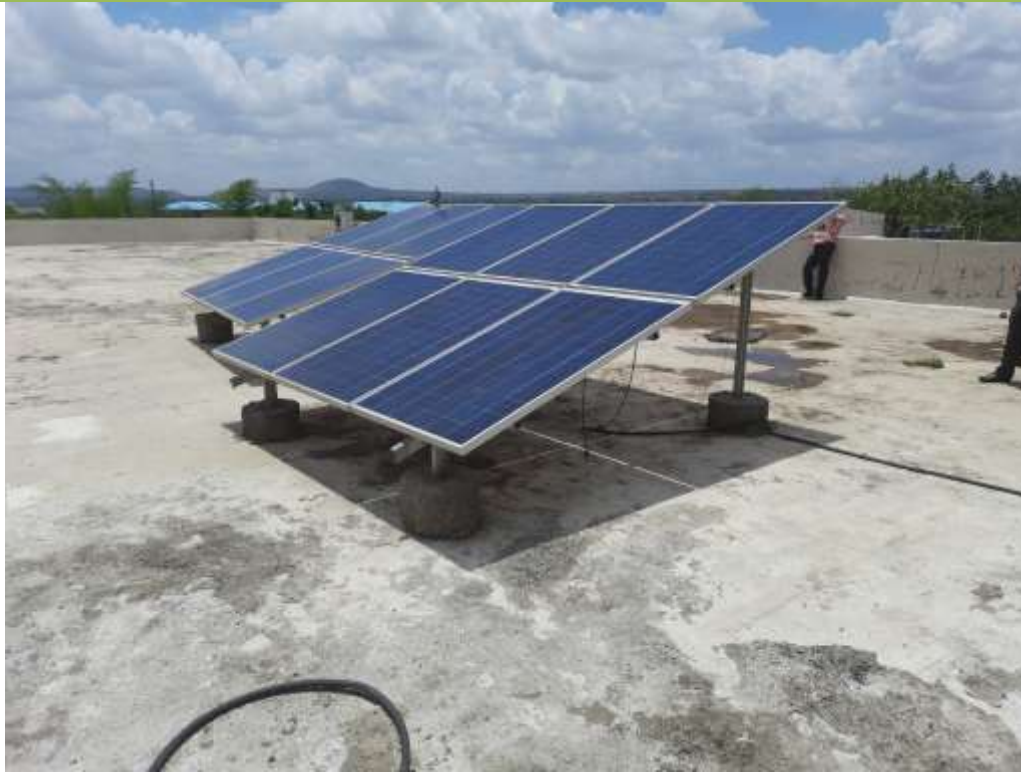
Solar Photovoltaic System- 3kWp- Admin building
