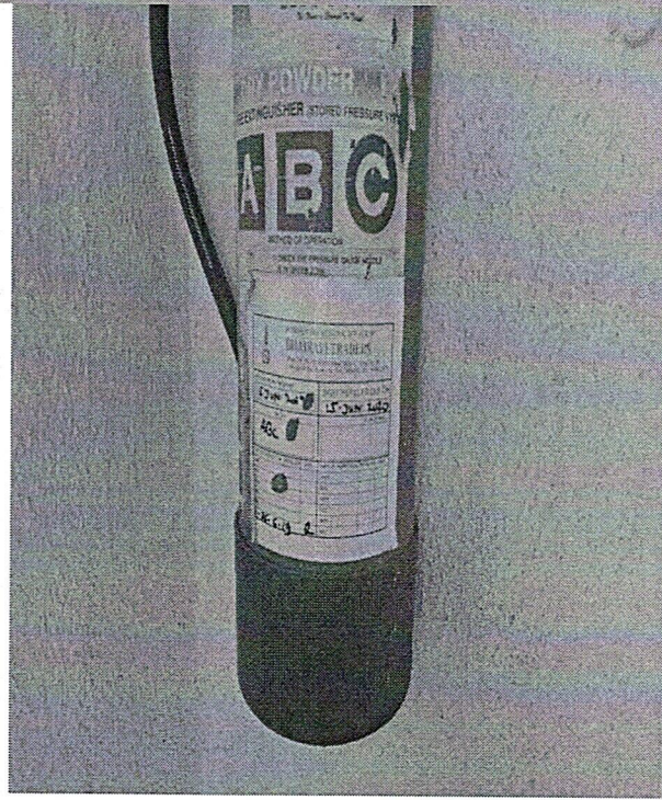
Validity of Fire extinguishers
