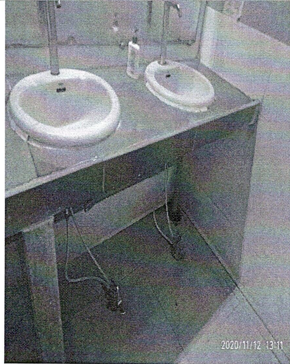
College can adopts hands free water taping system. This saves the water and also good for personal health protection to avoid frequent hand touching to water taps.
