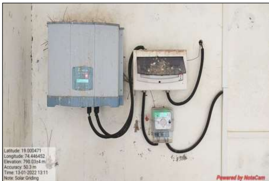
Picture 8: Solar Energy wheeled to grid panel at Administrative Building
