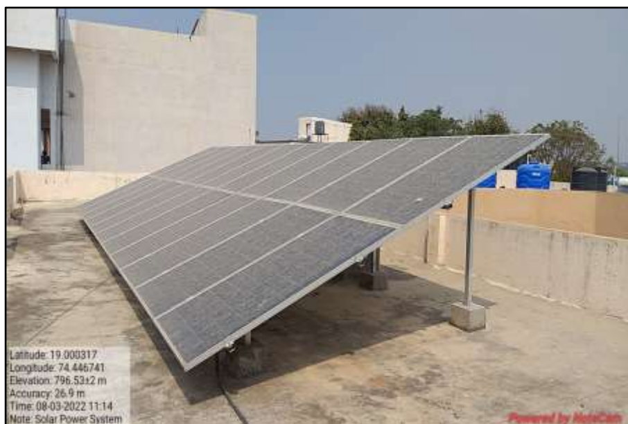
Picture 2: Solar Power System (Ladies Hostel)
