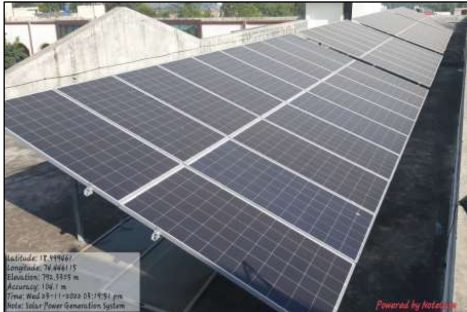
Picture 5: Solar Power System (Science Building)
