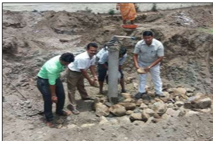
Picture 33: Laying of Stone Boulders around the around casing pipe in Excavation Pit
