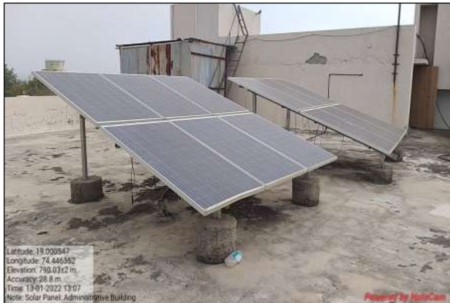
Picture 1: Solar Power System (Administrative Building)
