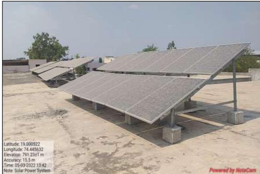
Picture 3: Solar Power System (Arts and Commerce Building)
