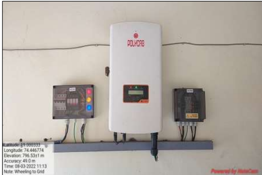
Picture 7: Solar Energy wheeled to grid panel at Rajmata Jijau Girl's hostel
