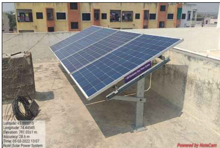
Picture 4: Solar Power System (Science Building)
