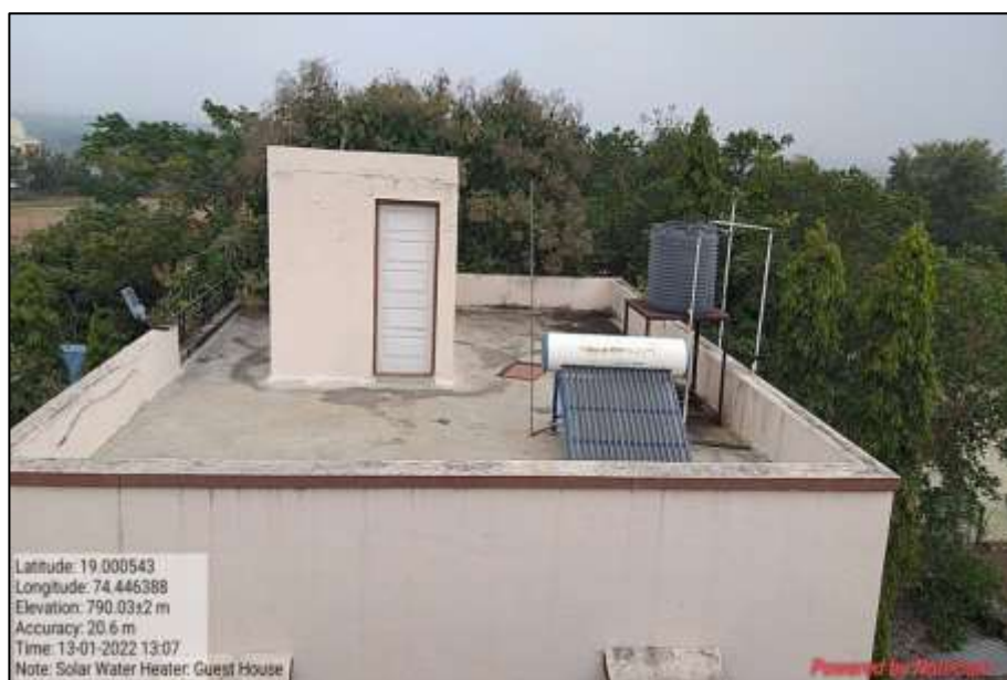
Picture 6: Solar water heater at Guest House
