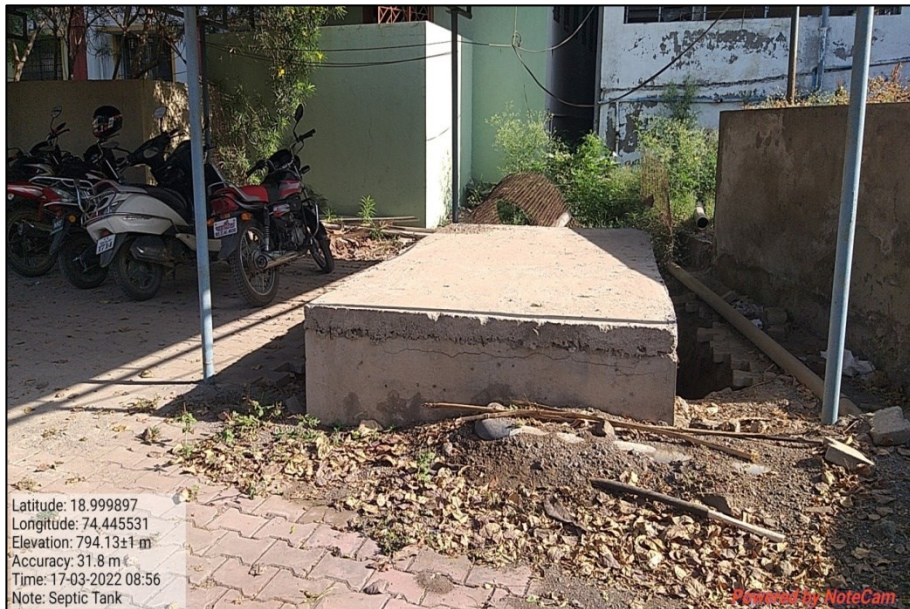
Picture 38: Septic Tank
