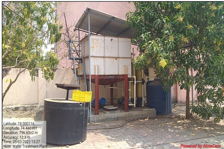
Picture 36: Waste Water Treatment Plant
