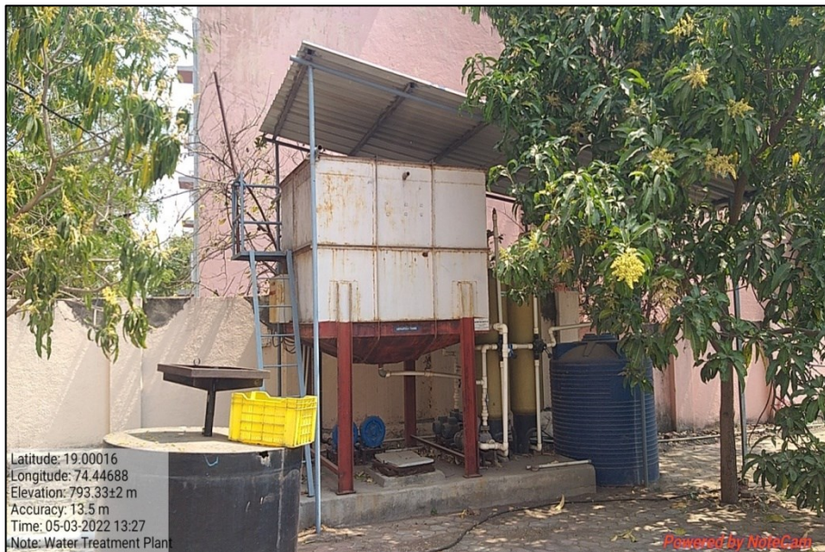
Picture 44: Waste Water Treatment Plant
