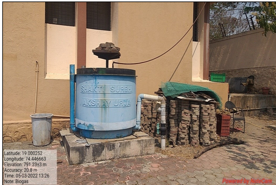
Picture 35: Biogas Plant at Rajmata Jijau Girl’s hostel
