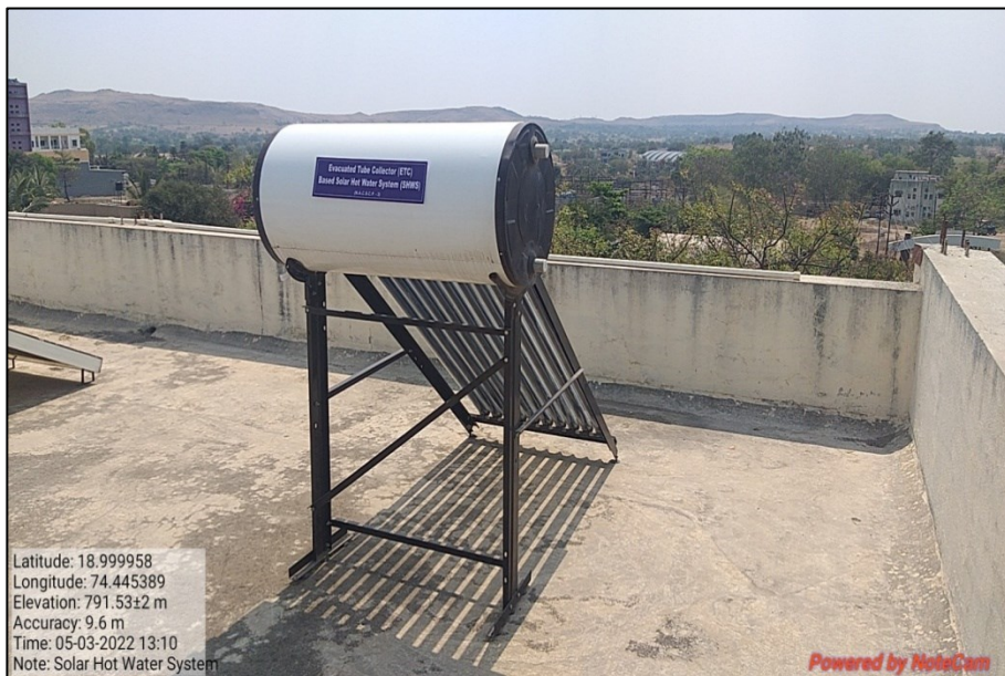
Picture 12: Solar water heater (ETC based) at Science Building
