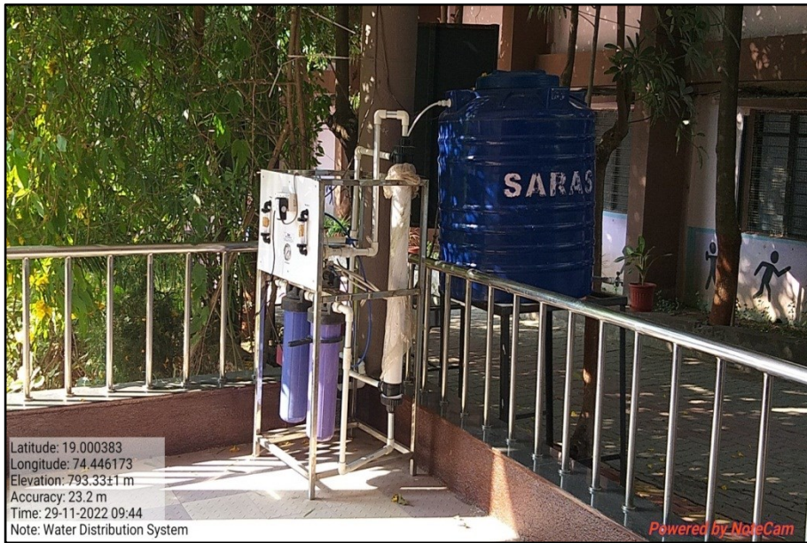
Picture 47: Water Purification System
