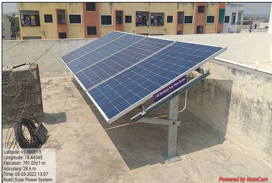
Picture 4: Solar Power System (Science Building)
