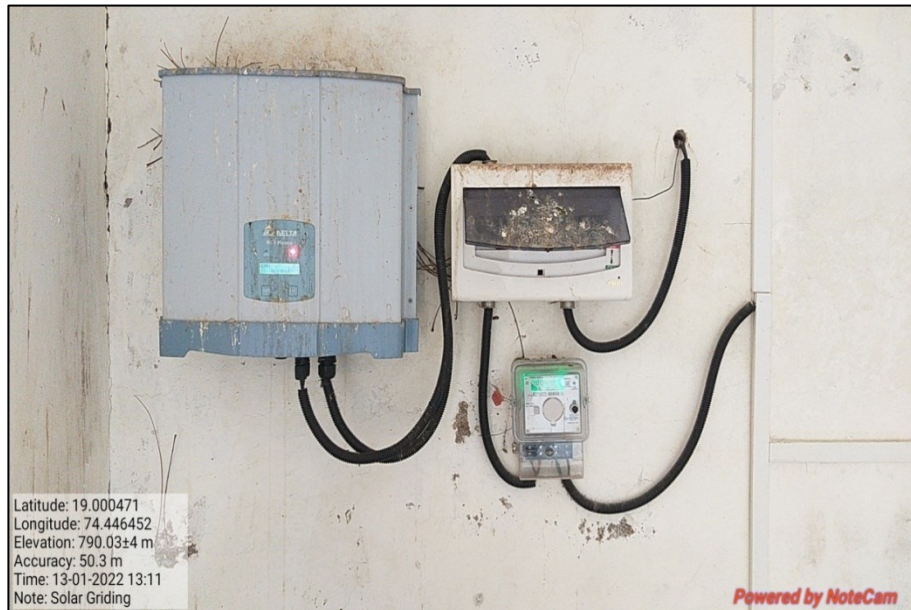
Picture 15: Solar Energy wheeled to grid panel at Administrative Building
