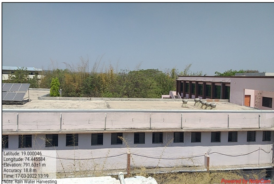
Picture 40: Rain Water Harvesting Pipes and Drain system
