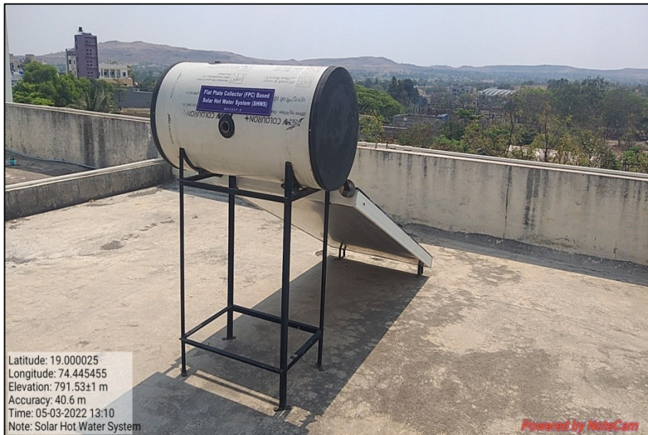
Picture 11: Solar water heater (FPC based) at Science Building
