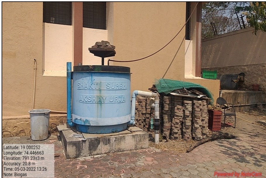
Picture 13: Biogas Plant at Rajmata Jijau Girl’s hostel
