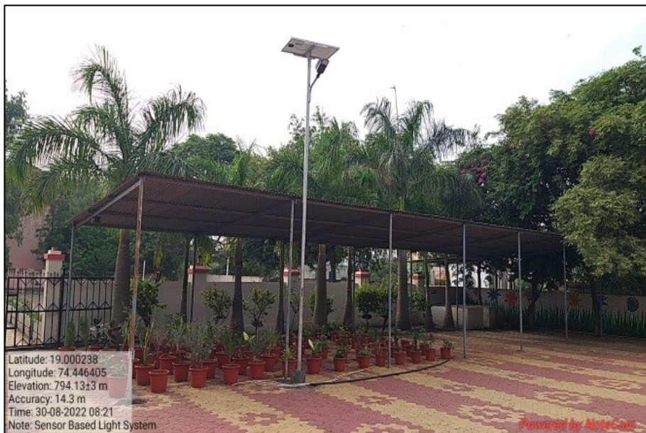
Picture 22: Sensor Based Energy Conservation through Street Lights
