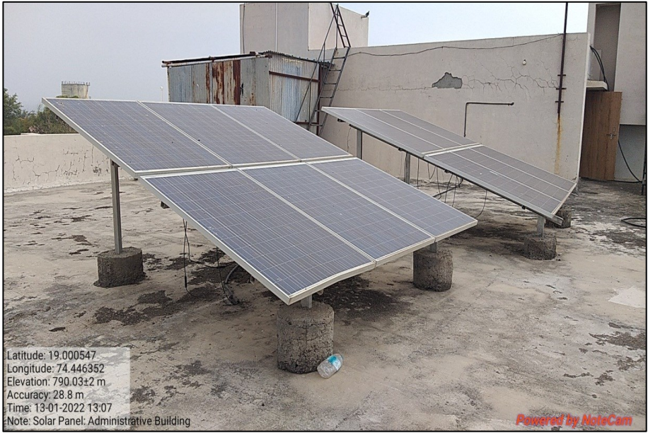
Picture 1: Solar Power System (Administrative Building)
