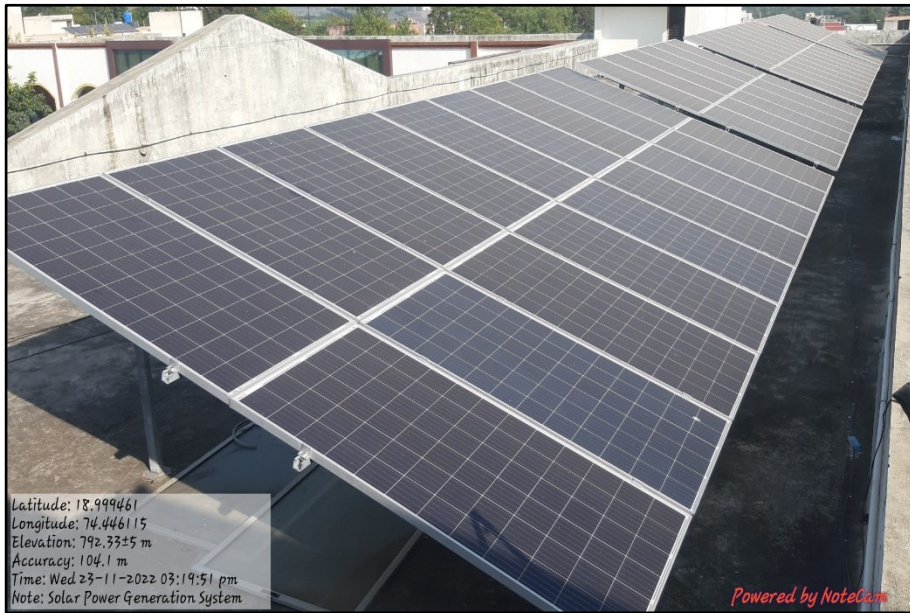
Picture 5: Solar Power System (Science Building)
