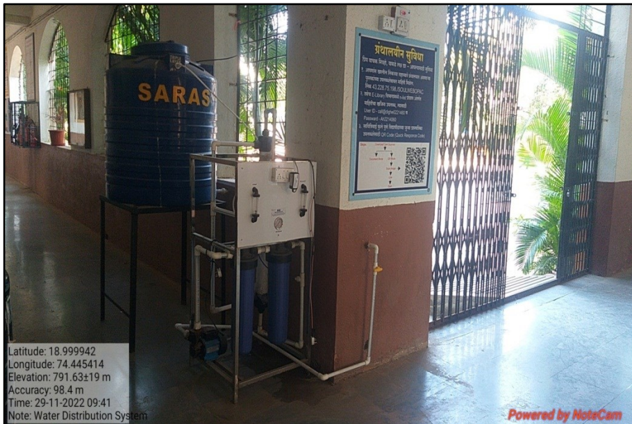
Picture 46: Water Purification System
