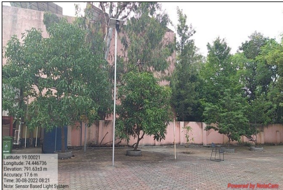
Picture 25: Sensor Based Energy Conservation through Street Lights
