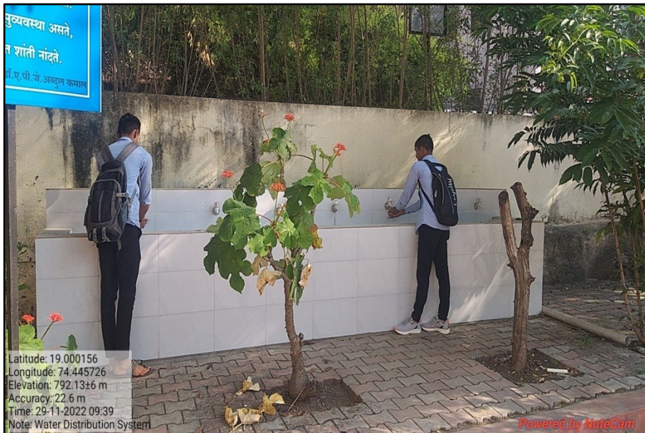
Picture 52: Water Distribution System
