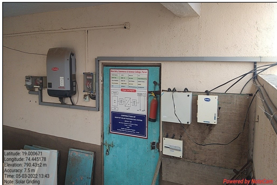
Picture 16: Solar Energy wheeled to grid panel at Arts and Commerce Building
