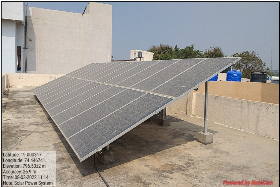
Picture 2: Solar Power System (Ladies Hostel)
