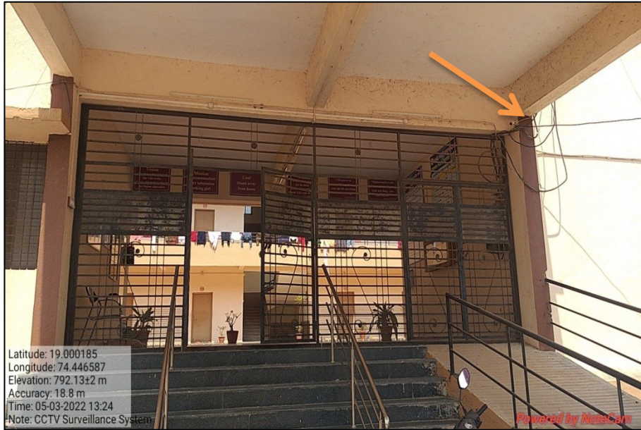
Picture 83: CCTV Surveillance System at Rajmata Jijau Girl’s hostel
