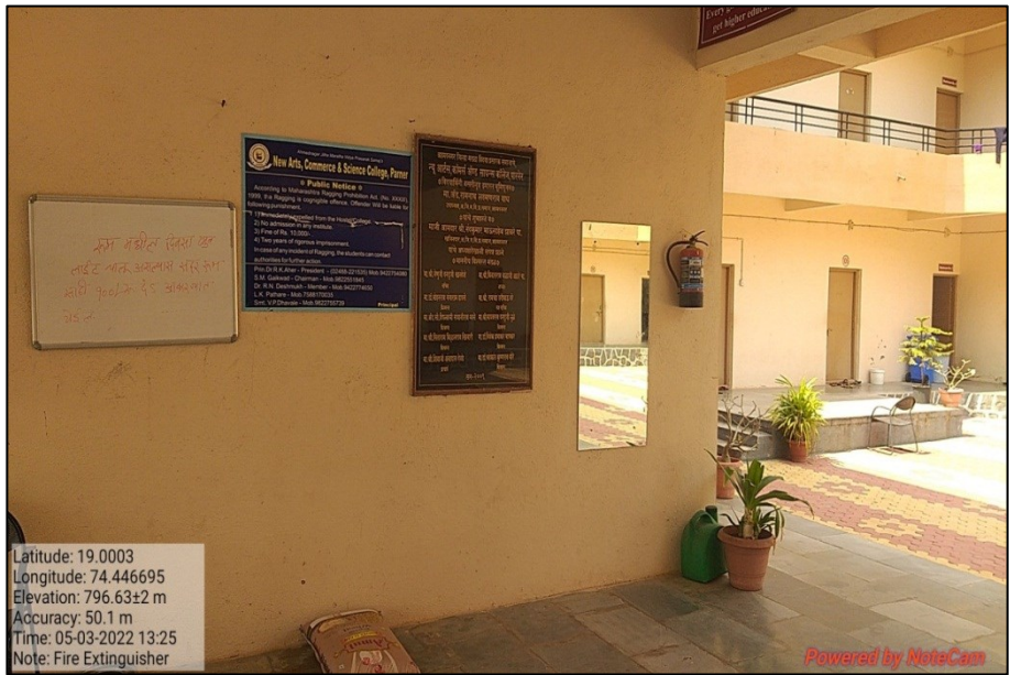
Picture 91: Fire Extinguisher at Rajmata Jijau Girl’s hostel
