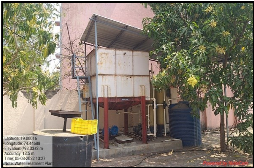
HTTP plant Infront of Ladies Hostel
