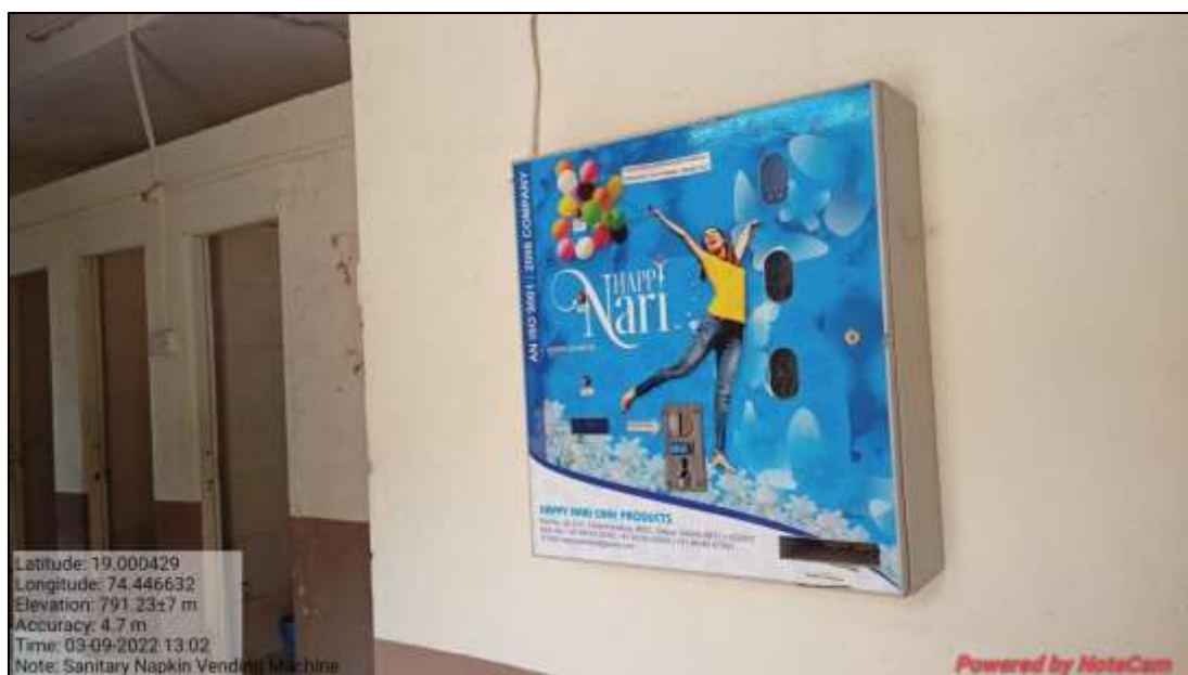
Figure 18: Sanitary Napkin Vending Machine in the Washroom Facility (Girls Hostel)
