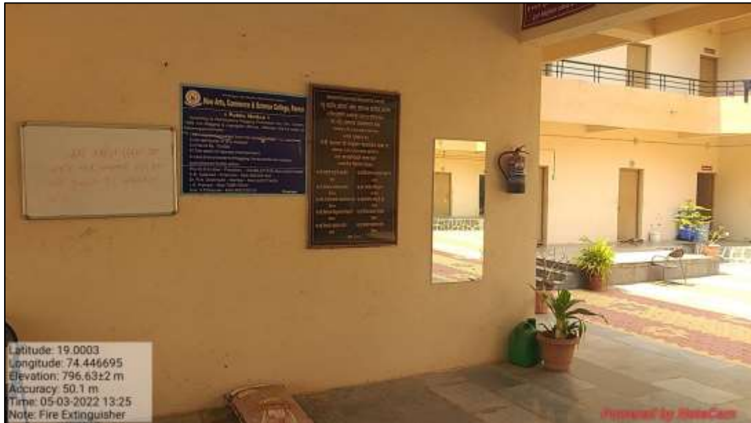
Figure 9: Fire Extinguisher at Rajmata Jijau Girl's hostel
